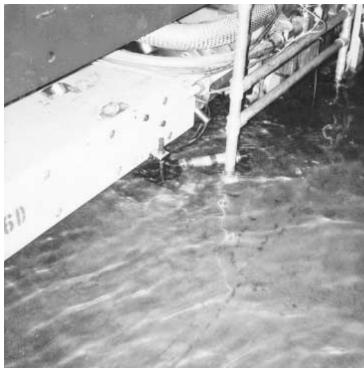
...to accumulate beneath Tevatron magnets in Main Ring tunnel.
