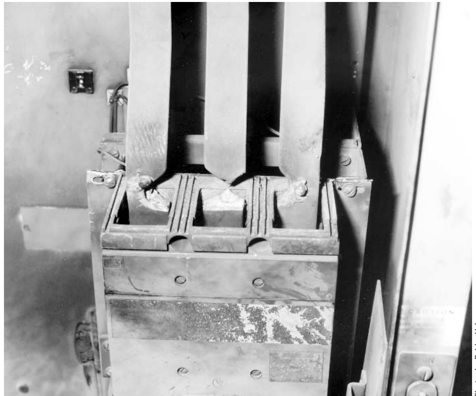
The motor control cabinet, where the electrical accident occurred.
