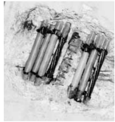
Post-tensioning cables originally were sheathed in hard plastic and encased in the concrete beams.
