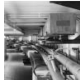
The Recycler, at the top of the photo, needs no power, cooling water, or fancy control systems to run.
